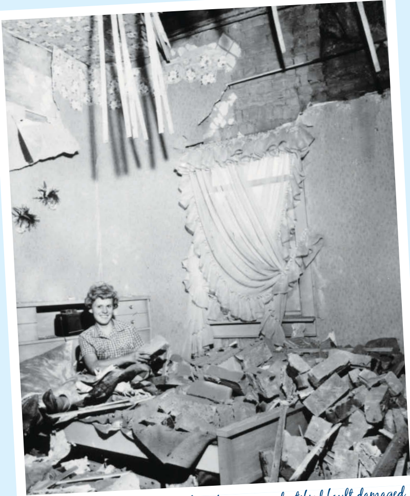
In 1962, a magnitude 5.7 earthquake on an unidentified fault damaged this bedroom in Richmond, Utah, a small town about 20 miles west of Bear Lake. A magnitude 7.4 earthquake (maximum expected for the eastern Bear Lake fault) would release approximately 80 times the energy and cause substantial damage, especially to historic structures. Photo courtesy of Ariel D. Benson, Richmond, Utah.
